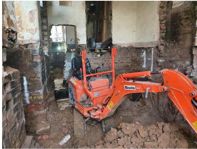
Figure 2: unauthorised excavation January 2021
