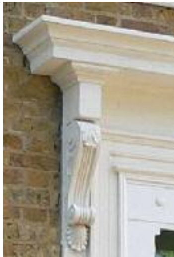
Consol bracket to window architrave, detail at No. 6 Aberdeen Terrace (left) and painted over at No. 5 (right).
