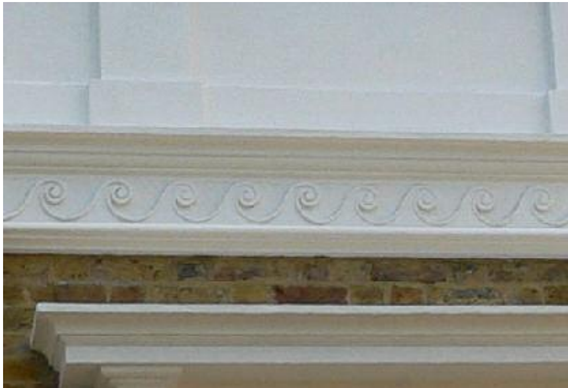
Stucco frieze with Terracotta Vitruvian scroll ornament painted over, detail at Aberdeen Terrace No. 5 (photograph taken 17.6.2009)
