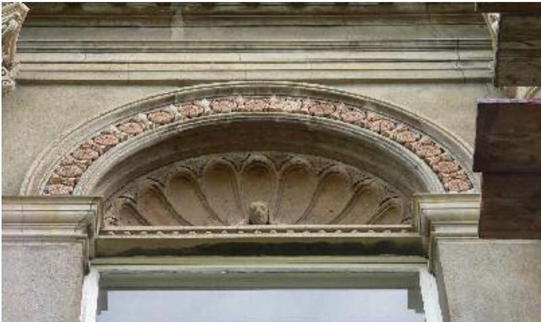
Stucco and Terracotta detailing of the fan moulding at the central bay to No. 6 Aberdeen Terrace (photograph taken 7.10.2010)
