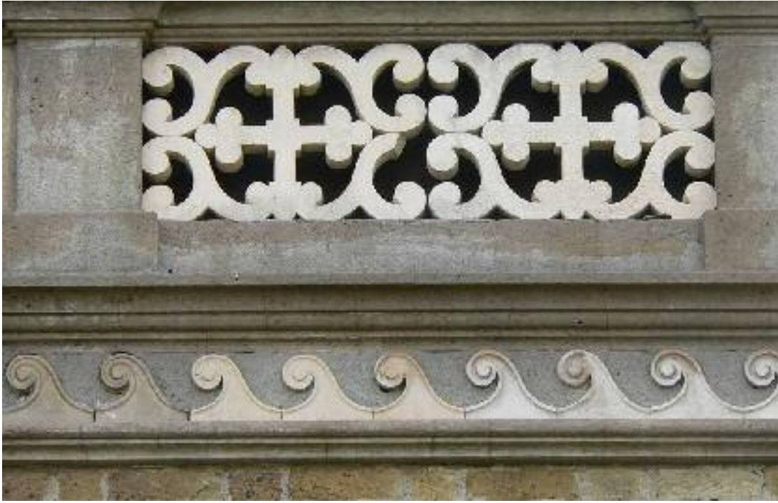
Stucco frieze with Terracotta Vitruvian scroll ornament and Terracotta balustrade above, detail at Aberdeen Terrace No. 6 (photograph taken 7.10.2010)
