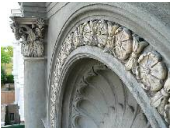
Terracotta Rosette frame surrounding the fan moulding at No. 4 Aberdeen Terrace (photograph taken 10.7.2010)
